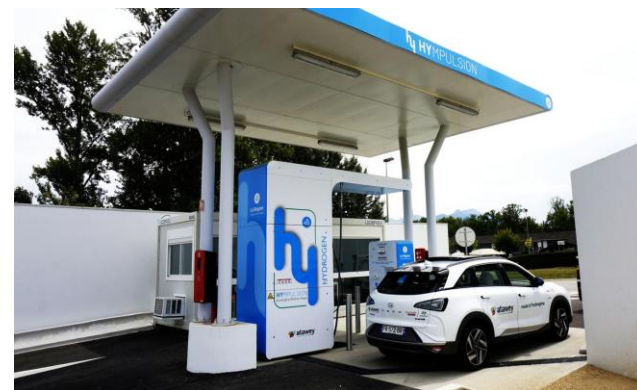
Station hydrogène (H2-mobile)
